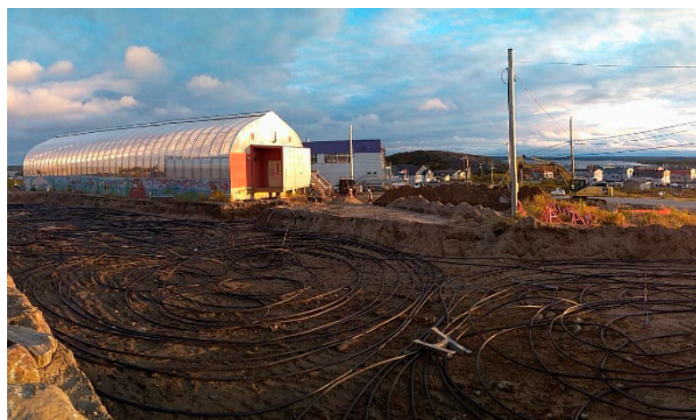
Figure 11. Kuujuaq, Quebec: geothermal pilot project, 30 kW horizontal GHSP system for the community's swimming pool.
